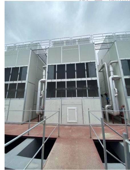
IEC water chillers
