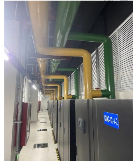
Air conditioning boxes
